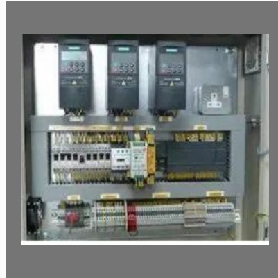
AC Drive control panel
